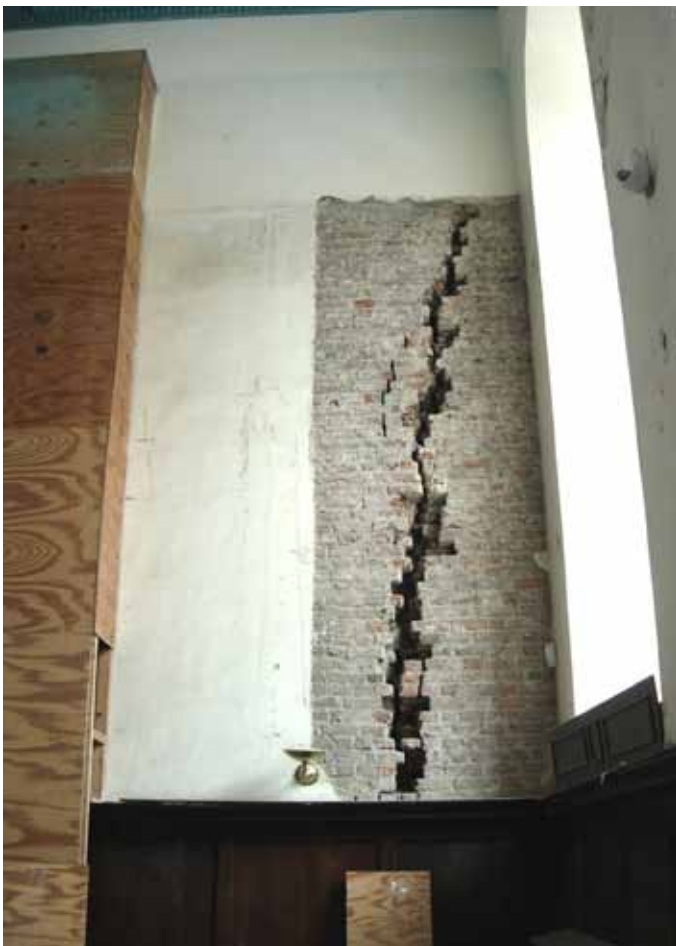
Large structural crack through existing wall
